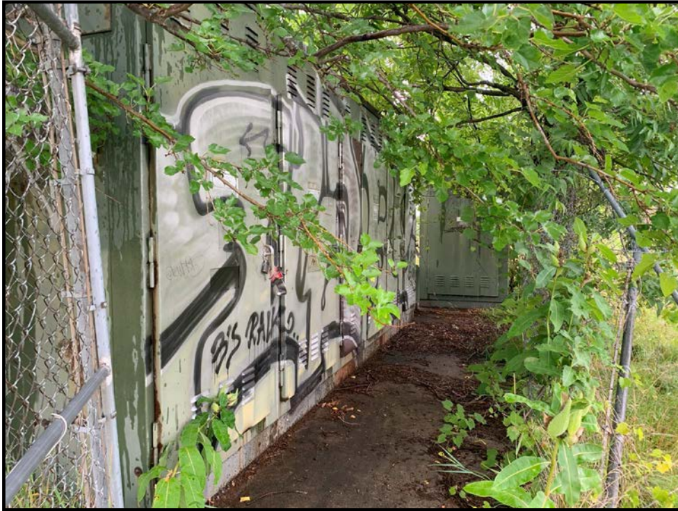
Photo 5: View of the electrical utility on the southwestern portion of the subject property.
